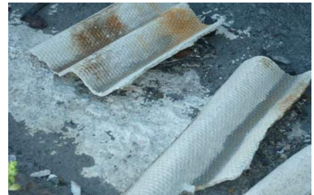
Asbestos Sheeting (Ian Murgatroyd)
